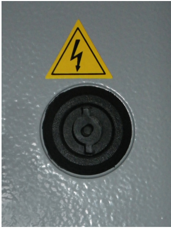
Control cabine locks to keep unauthorized personnel out.
